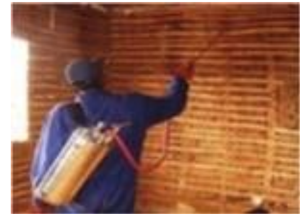
Indoor Residual Spraying (IRS)
